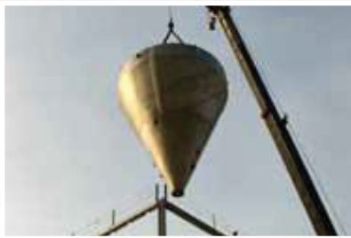
Left: Large capacity spray drying plant installation. Spray dryer delivered to site in sections for final fabrication.
